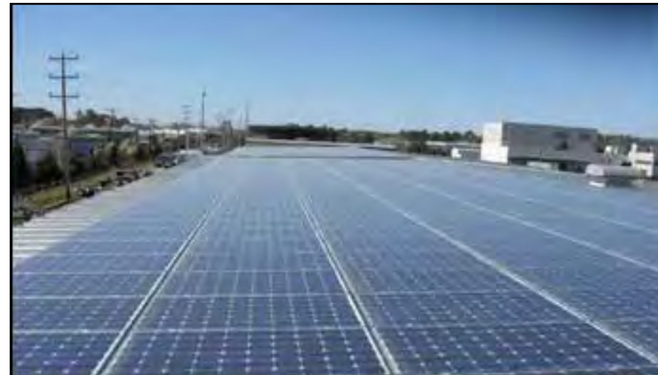
Solar Array on Santee Cooper Facility Source: Santee Cooper
