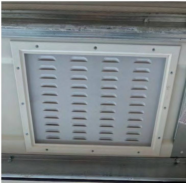
NON-ENGINEERED FLOOD VENT IN GARAGE DOOR
