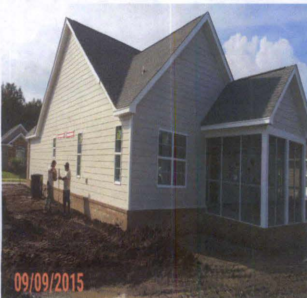
Right side HVAC Rear
