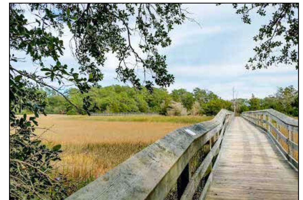
Vereen Memorial Gardens Boardwalk needs repair
