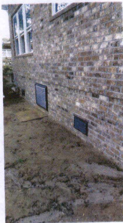
LARGE VENT AND SMALL VENTS
