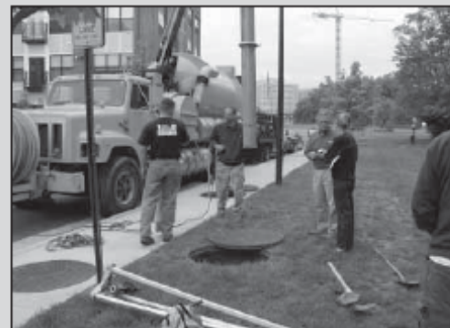
A vacuum truck may be required to remove sediment from stormwater facilities located underground.
