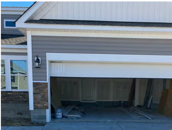
NON-ENGINEERED FLOOD VENT IN GARAGE DOOR
