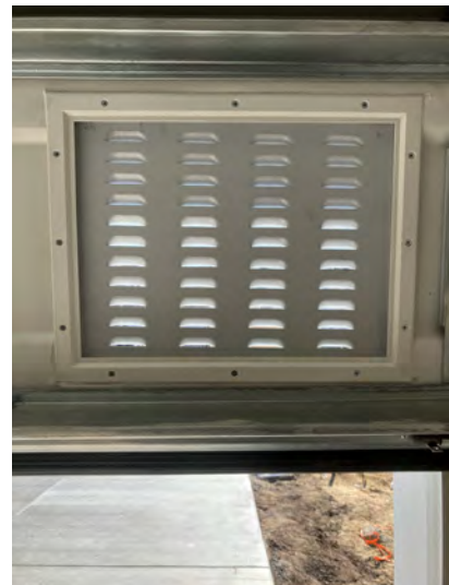
BACK OF NON-ENGINEERED FLOOD VENT
