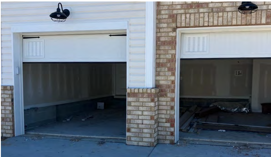
NON-ENGINEERED FLOOD VENTS IN GARAGE DOOR
