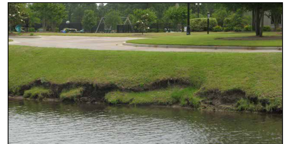
Pond Bank Erosion Photo Credit: Clemson Extension
