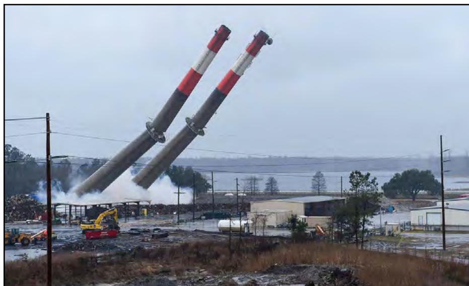
Demolition of the Granger Generating Station stacks Photo Credit: Jim Huff, Santee Cooper
