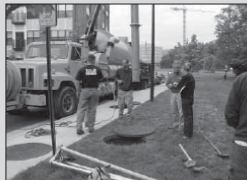
A vacuum truck may be required to remove sediment from stormwater facilities located underground.
