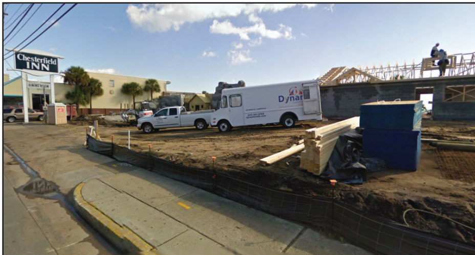
The site of the Chesterfield Inn being developed into a strip mall Source: Google
